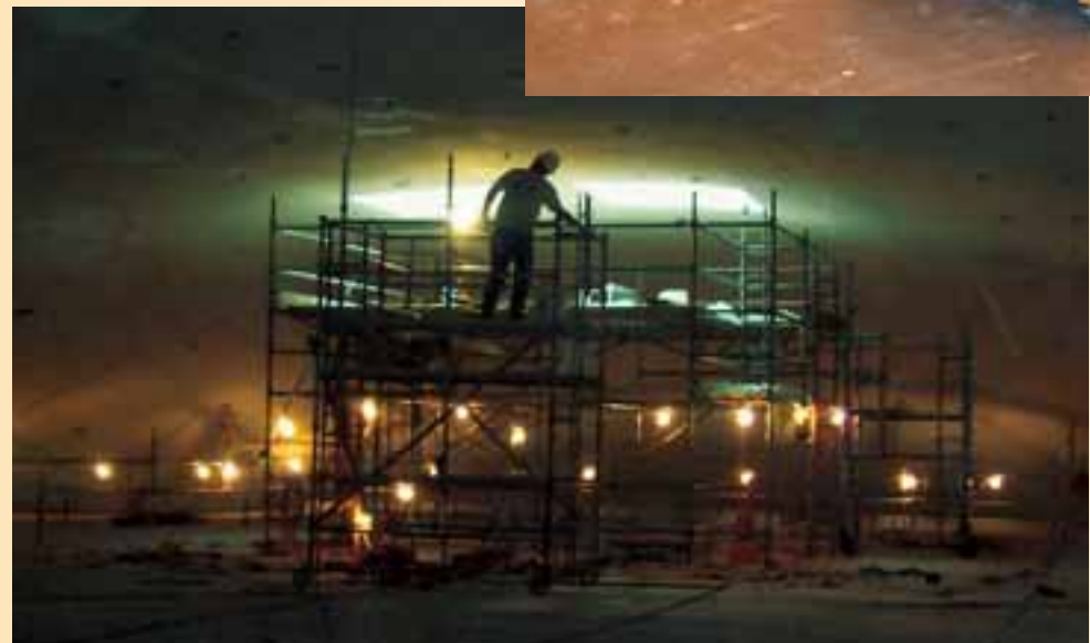
A worker stands atop scaffolding that is several stories high as he works on the restoration of the ceiling. Fourteen layers of paint were removed to reach the original plaster. After repairs were made, workers applied plaster that matched the properties of the historic plaster in both its content and acoustic properties. Care was taken to preserve the waviness of the original ceiling.
