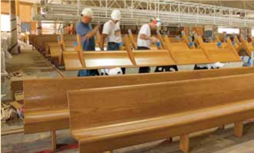
Above: Workers install solid white oak pews , which will replace most of the original soft pine ones. The original pews, painted by pioneer artisans to look like oak, were damaged and worn. Some will be permanently displayed.
