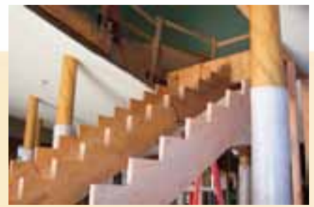
One of two new staircases added to the balcony makes six exits from the upper floor.
