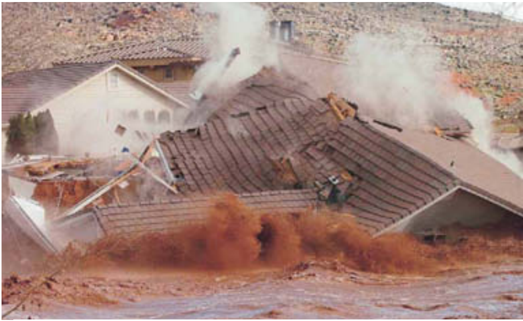
A St. George, Utah, home collapses into floodwaters that ate away the home's foundation.
