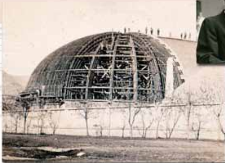
Above: Workers atop the building completing construction of the roof on the west end of the Tabernacle. Above center: President David O. McKay at the pulpit with Elder Spencer W. Kimball in the background. Right: Exterior view of the Tabernacle dome and the spires of the Salt Lake Temple.
